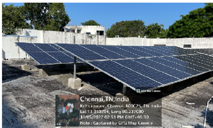
Power generation through Solar PV Panels
